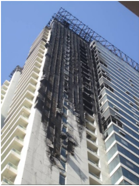
Picture-2 Façade Fire at Tamweel Tower.
