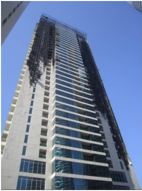
Picture-3 Façade Fire at Tamweel Tower.
