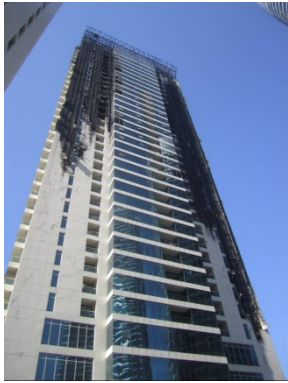
Picture-3 Façade Fire at Tamweel Tower.
