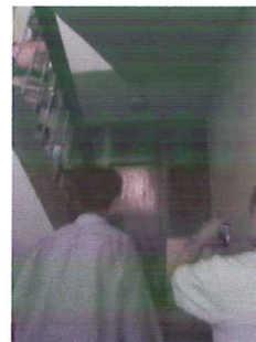
Picture-9 Sole staircase without vertical compartment.
